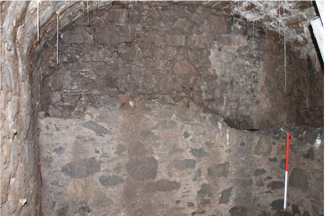
Plate 1: Main chamber, general view of the west wall showing the inner skin wall, from the SEE
