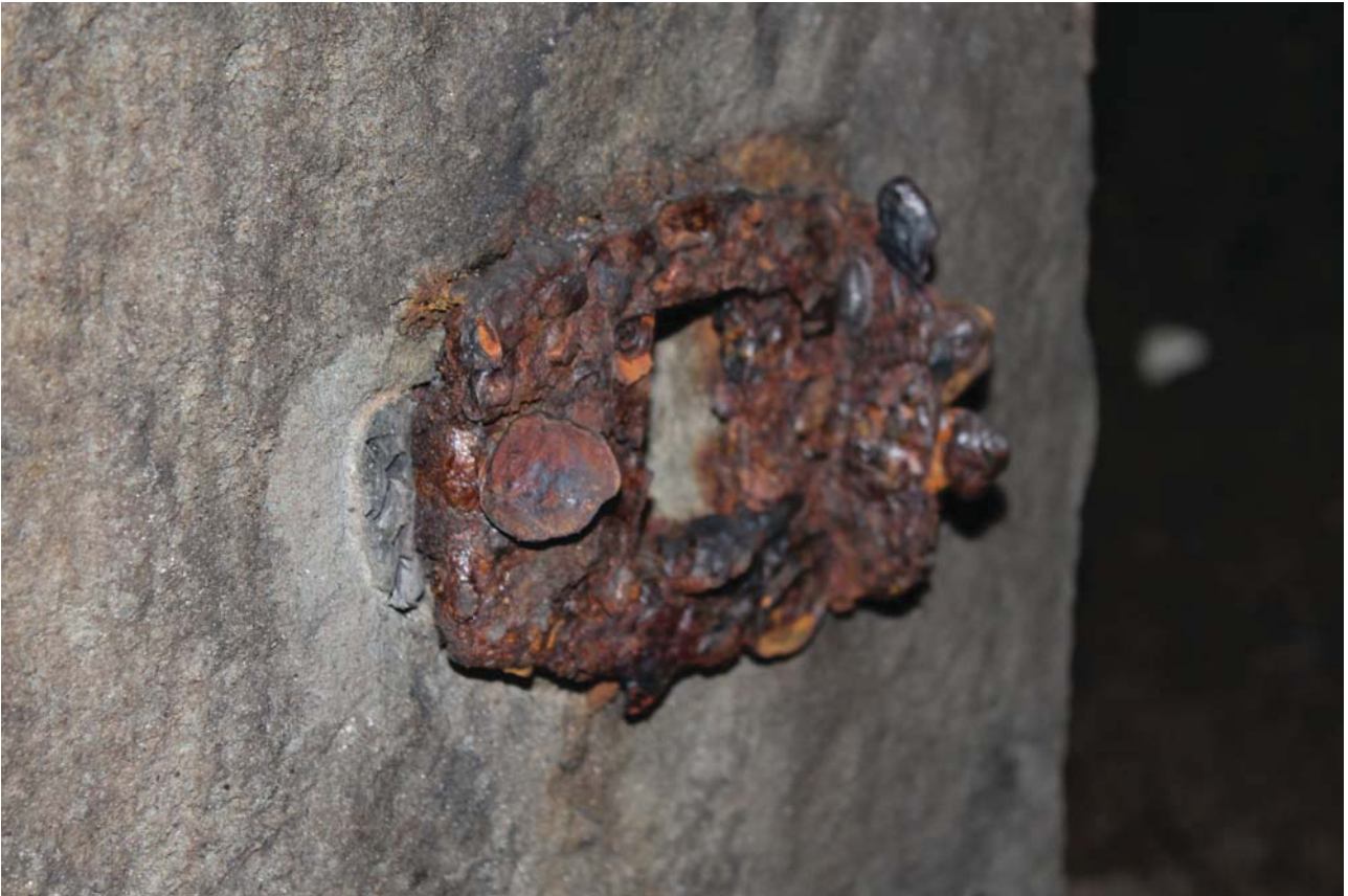
Plate 7: Former gated entrance, detail of rusted fitting in the west side, from the north-west
