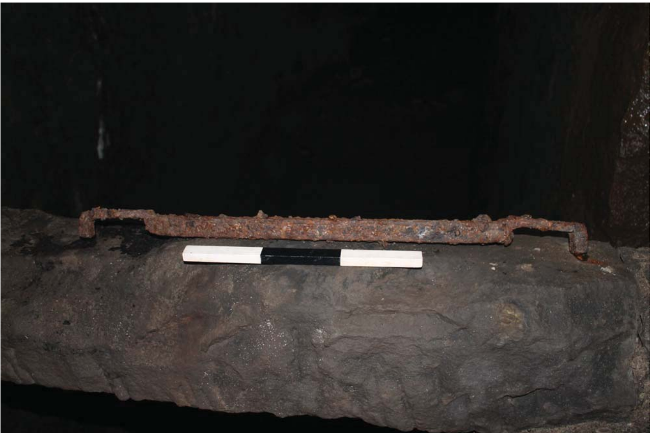
Plate 8: Former gated entrance, detail of rusted iron latch, from the south-east
