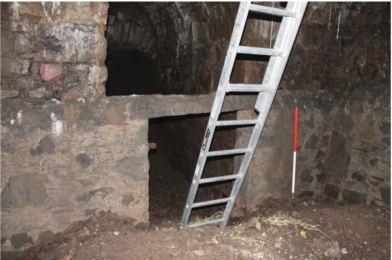
Plate 4: Main Chamber, general view of the north inner skin wall showing the main former gated entrance, from the south-west
